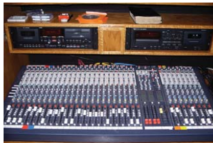
A Soundcraft LX7ii 32-channel mixing console the centerpiece of the AV system at Lake Grove Missionary Church in Memphis, TN
